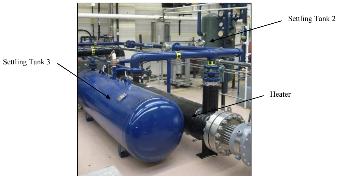
Figure 2.3: Settling tank 2, settling tank 3, and heater.
